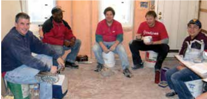
Volunteers from Dow have been a key part of the rehabilitation of this home in Norristown, Pa., by Habitat for Humanity of Montgomery County. Pictured: Jim Alexander, Stewart Williams, John Reffner, Marcelo Figueira, and Wei Gao.
