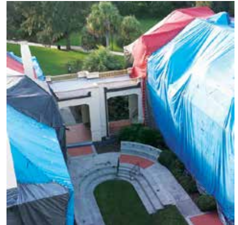
The Thomas Center is carefully tented during its fumigation by Southern Fumigation.
